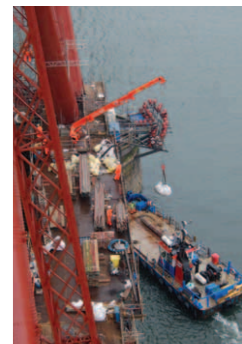
Loading of scaffolding materials onto barge at the Inchgarvie storage platform © John Andrew
