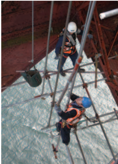
Scaffolders were employed to construct and remove the complex systems © Balfour Beatty
